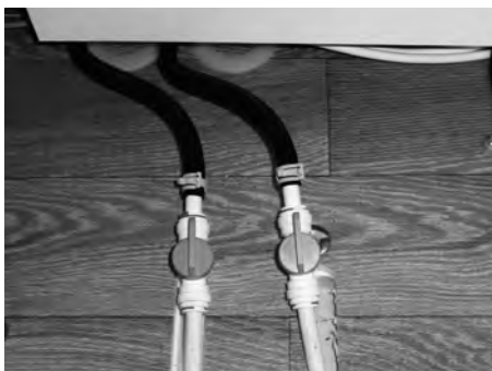
Ventile in offener Position
