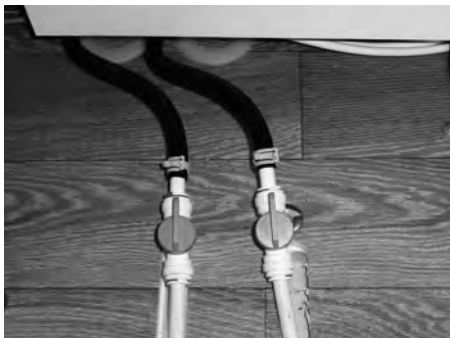
Ventile in offener Position
